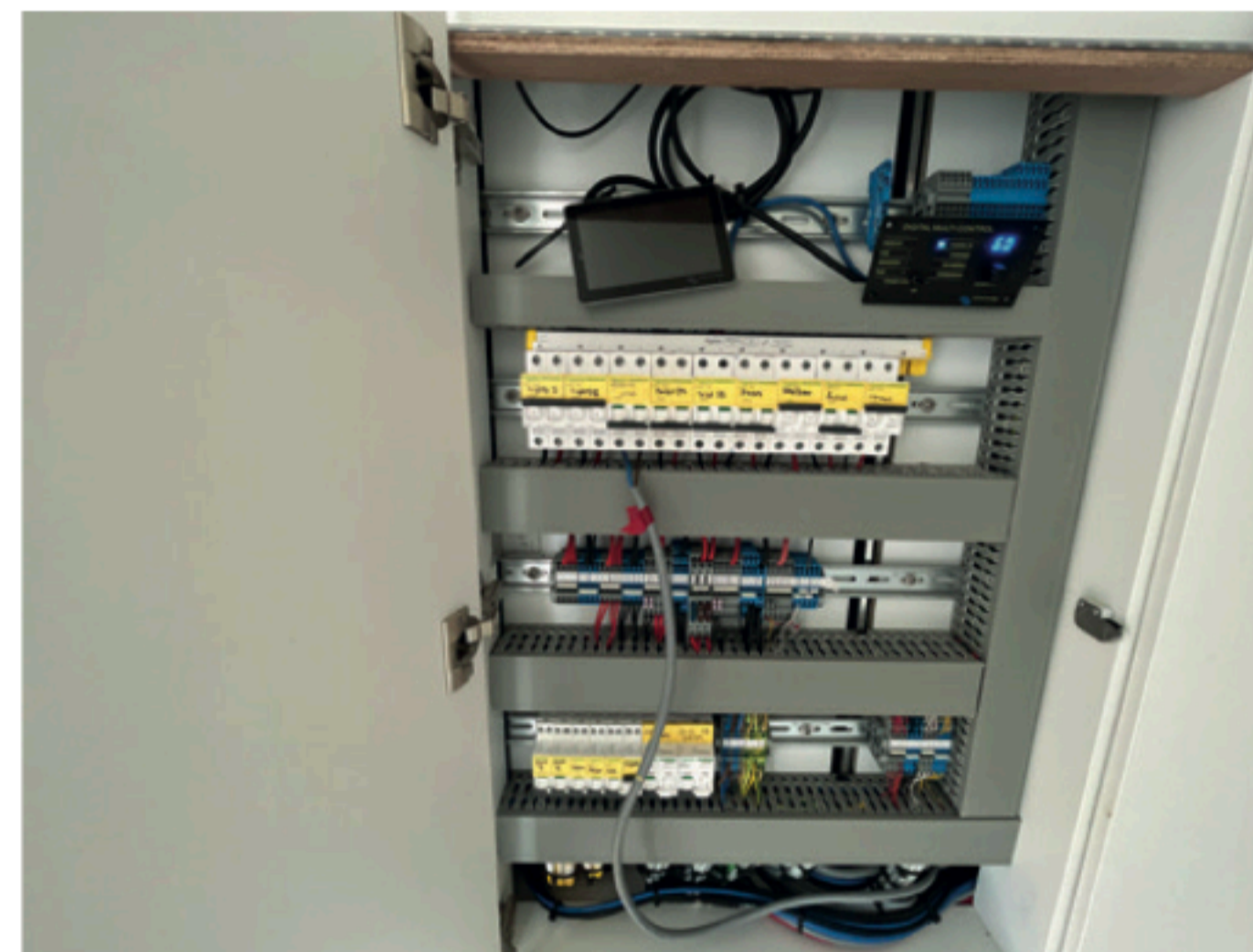
The electrical panels are easily accessible in the starboard hull.
